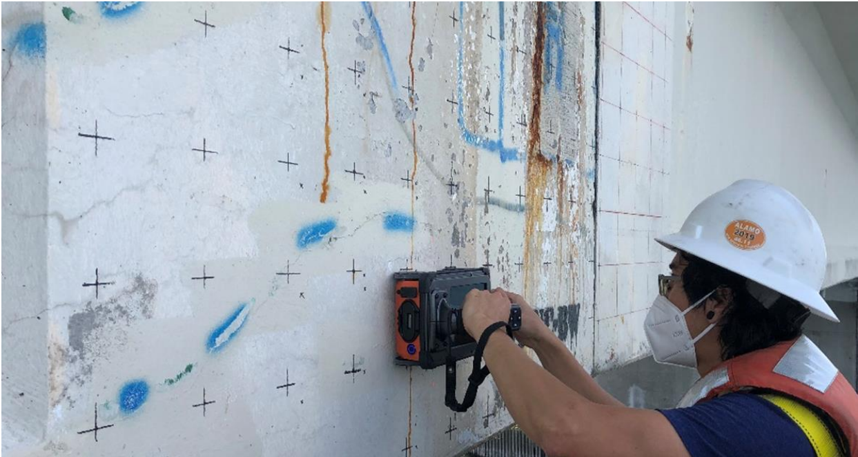
Figure 3: Horizontal GPR scanning on a 3 in (75 mm) grid (vertical scans were also completed) for 3-D GPR image
