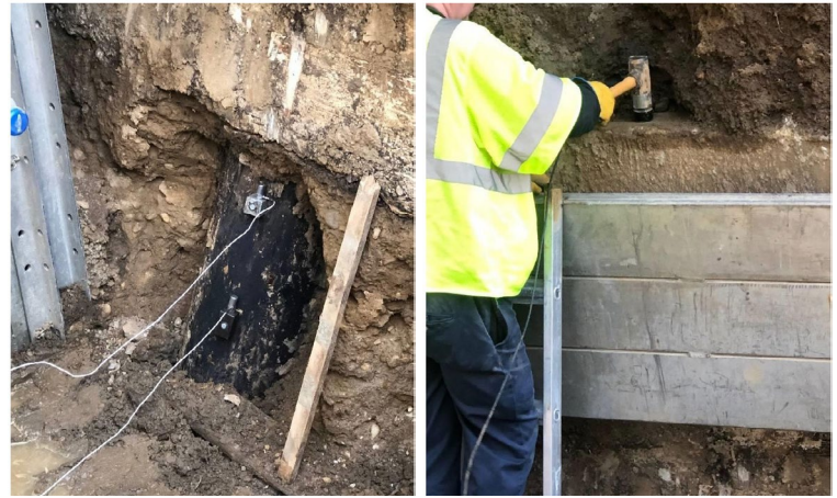
Figure 5. SE/IR testing on timber pile – left photo shows 2 accelerometer receivers mounted on blocks with wood lag bolts on the timber pile side at 4.5 and 5.5 ft below the top of the concrete pile cap. The right photo shows the 3 lb instrumented impulse hammer impacting the 4 ft thick concrete pile cap directly over the timber pile.
