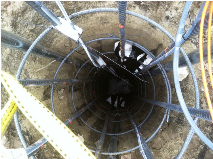
Figure 9. CSL and CT test shaft with sand bag defects that were installed at known depths prior to concrete placement.
