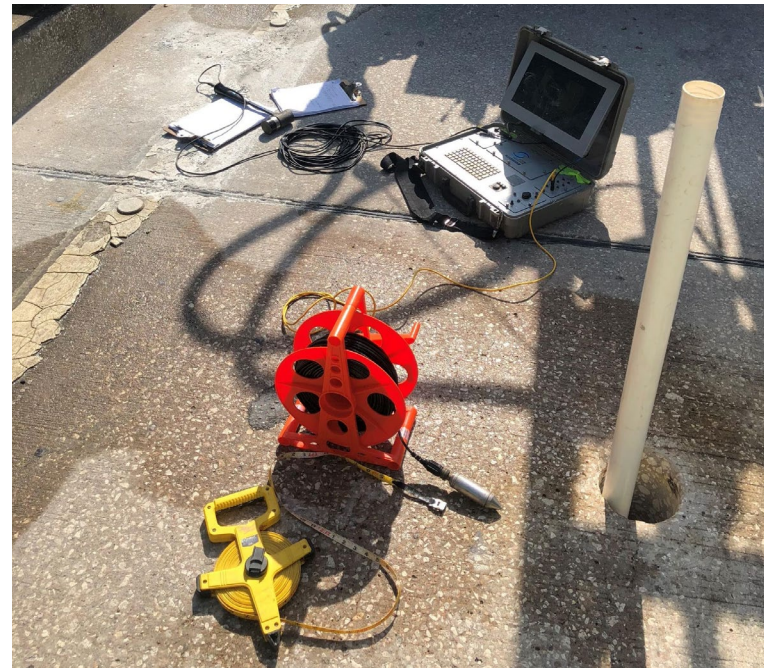
Figure 2 – Parallel Seismic (PS) test setup on a bridge deck with 3 lb impulse hammer, PC data acquisition system, hydrophone receiver and PVC boring casing filled with water.
